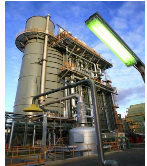
Gas fired cogeneration plant
