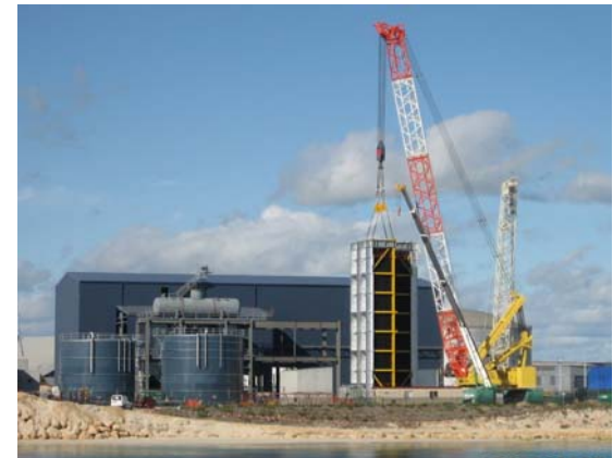
NewGen Kwinana combined cycle gas-fired power station
