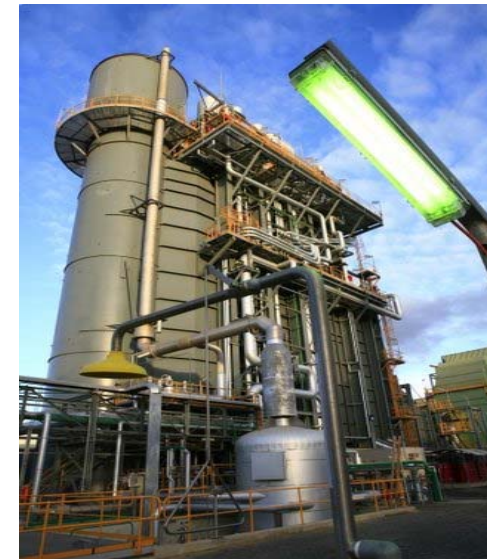
Gas fired cogeneration plant
