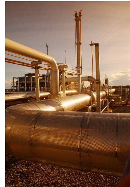
Dampier Bunbury Pipeline
