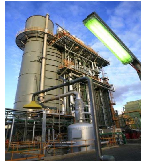
Gas fired cogeneration plant
