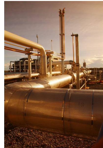
Dampier Bunbury Pipeline
