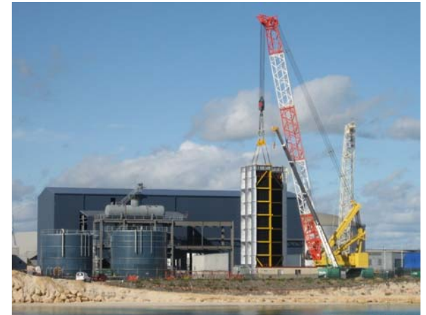
NewGen Kwinana combined cycle gas-fired power station
