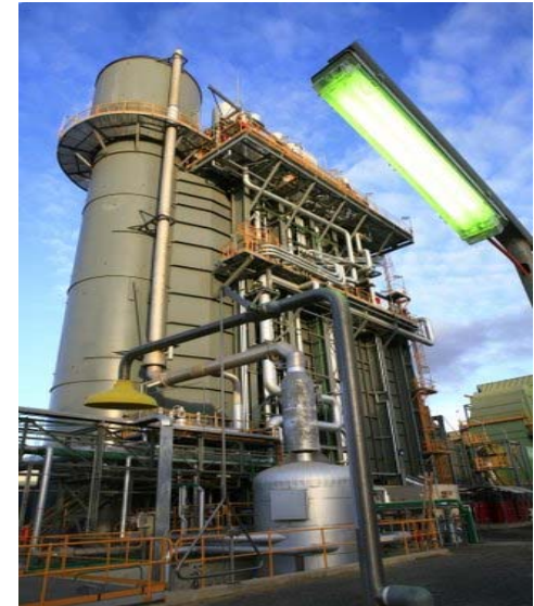
Gas fired cogeneration plant
